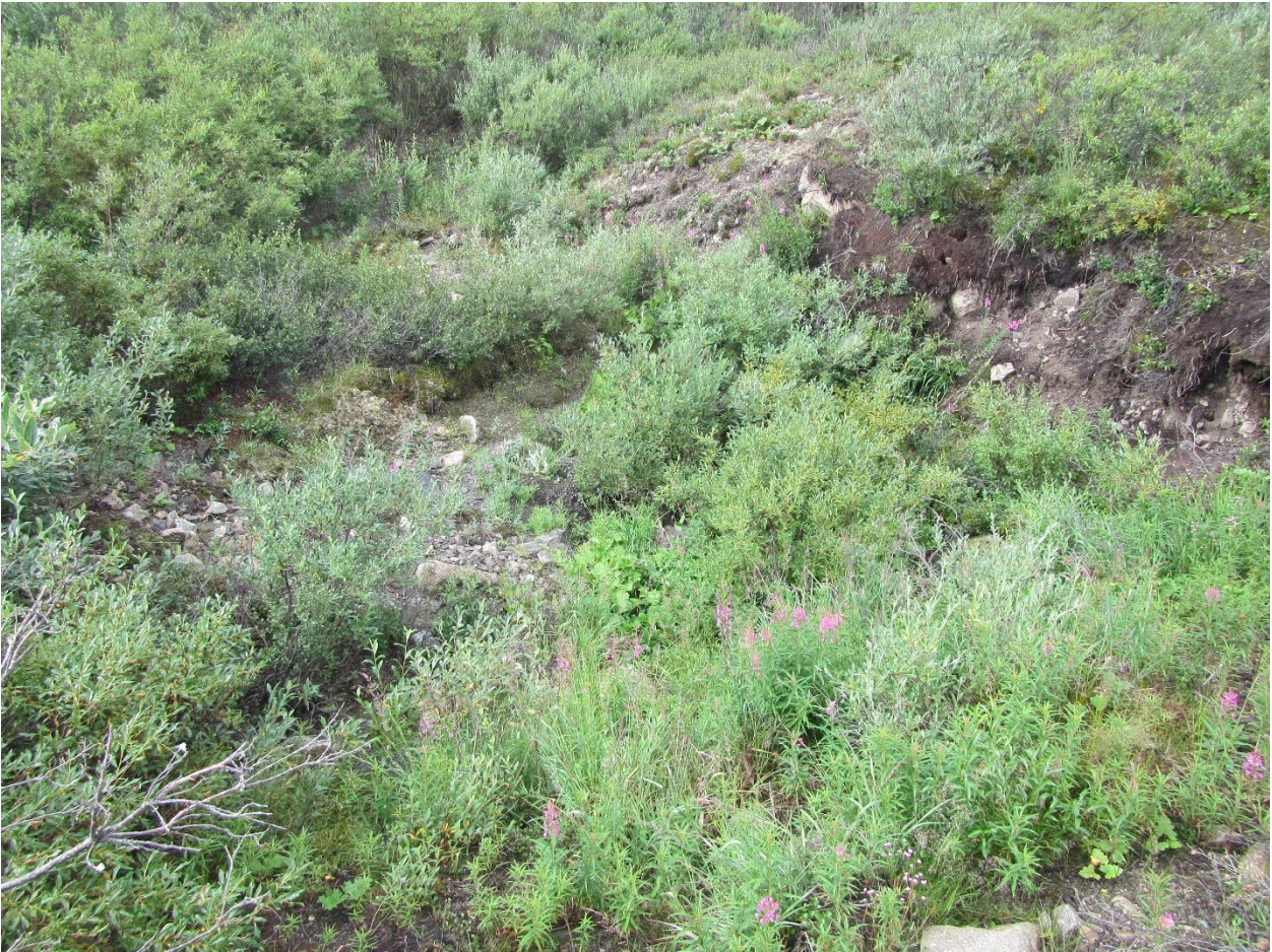
Figure 5.2. Depressed area with collapsing at the LHS.
