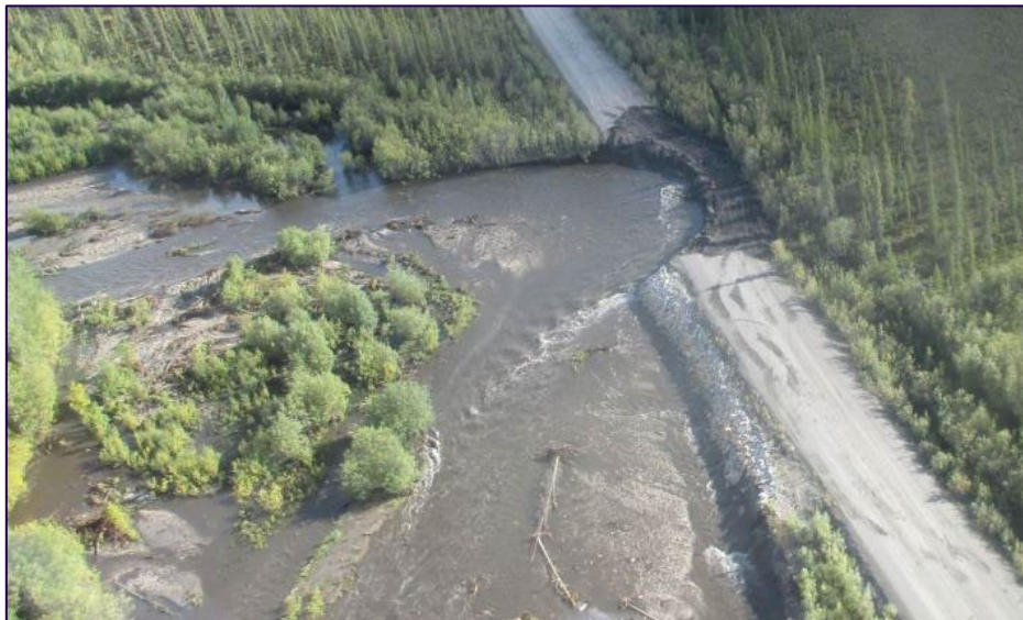
FIGURE 2.4. EROSION OF THE DEMPSTER HIGHWAY EMBANKMENT AT KM 166.5 FOLLOWING A HIGH-INTENSITY, MID-SUMMER RAIN EVENT IN AUGUST 2016 (PHOTO CREDIT: HPW).
