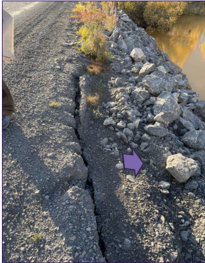
FIGURE 6.4. NEWLY INSTALLED RIPRAP AT DEMPSTER HIGHWAY KM 193.4 WAS LIKELY NOT SUFFICIENTLY EMBEDDED, WHICH HAS CAUSED TENSION CRACKS AND THE RIPRAP TO ‘SLIP’ DOWNWARD BY APPROXIMATELY 25 CM.
