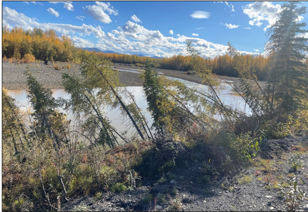
FIGURE 6.10. AN ERODING BANK OF OGILVIE RIVER IS WITHIN A FEW METRES OF THE ROAD EMBANKMENT AT DEMPSTER HIGHWAY KM 239.5 (PHOTO CREDIT: SLR, 2025). THE NEXT SIGNIFICANT HYDROLOGICAL EVENT MAY LEAD TO A ROAD WASHOUT.
