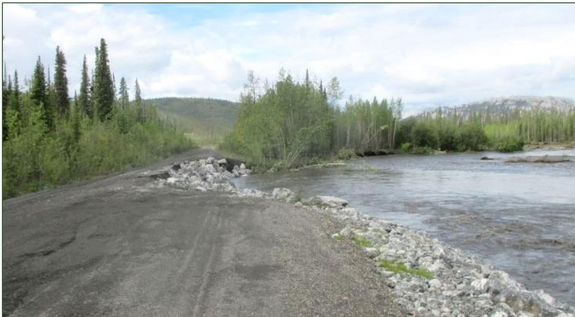
FIGURE 6.7. TEMPORARY EROSION MITIGATION FOLLOWING A ROAD WASHOUT AT DEMPSTER HIGHWAY KM 180.3 DURING THE AUGUST 2016 FLOOD (PHOTO CREDIT: HPW). THE TEMPORARY MEASURE DOES NOT NEGATE THE NEED TO RECONSTRUCT THE HIGHWAY, BUT IT MINIMIZES THE SERVICE DISRUPTION BY ALLOWING ALTERNATING TRAFFIC TO PASS UNTIL THE HIGHWAY IS RECONSTRUCTED.
