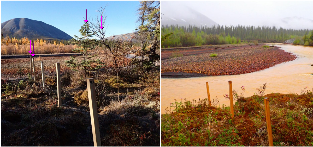
FIGURE 5.4. LEFT BANK OF ENGINEER CREEK IN SEPTEMBER 2024 (LEFT) AND JUNE 2026 (RIGHT) SHOWING THE LOSS OF TWO WOOD STAKES (PINK ARROWS) LOCATED AT DISTANCE 0.0 AND 1.0 M FROM THE BANK EDGE. THAT BANK RECEDED BY 2 M (STAKE 2.0 M WAS AT THE NEW BANK EDGE) IN 1.5 YEARS. PICTURES WERE TAKEN DURING SITE VISITS BY YUKONU AND ALSO REVEAL THE LOSS OF TWO SMALL TREES (OTHER PINK ARROWS).
