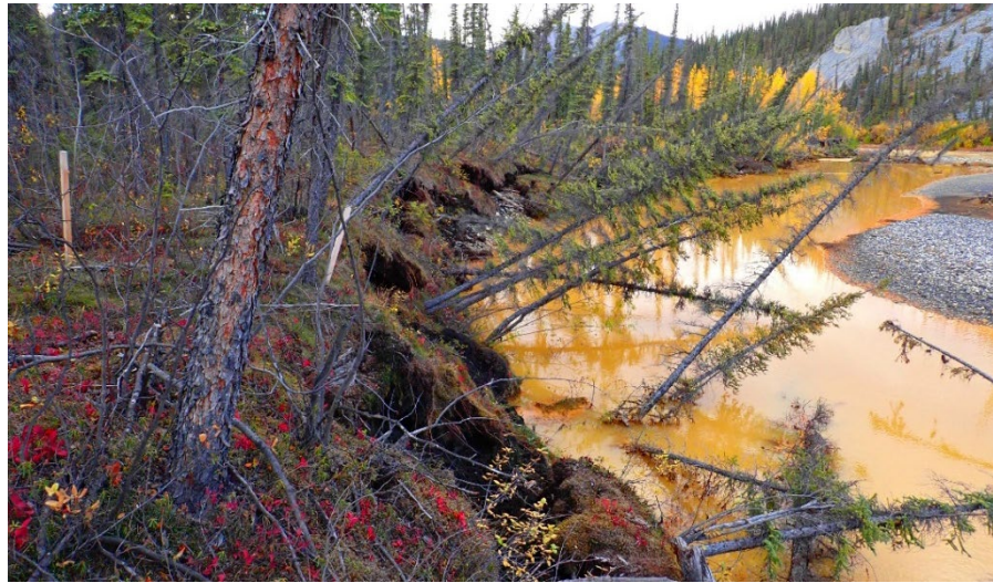
FIGURE 5.2. DOWNSTREAM VIEW OF KM 194.0 SHOWING SEVERAL TREES THAT ARE GRADUALLY FALLING INTO ENGINEER CREEK (SEPTEMBER 2025).
