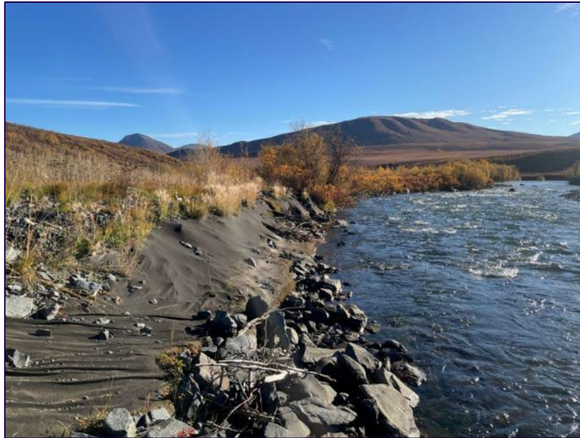
FIGURE 6.1. RIPRAP HAS BEEN DISPLACED ATOP GEOTEXTILE AT DEMPSTER HIGHWAY KM 107.8.
