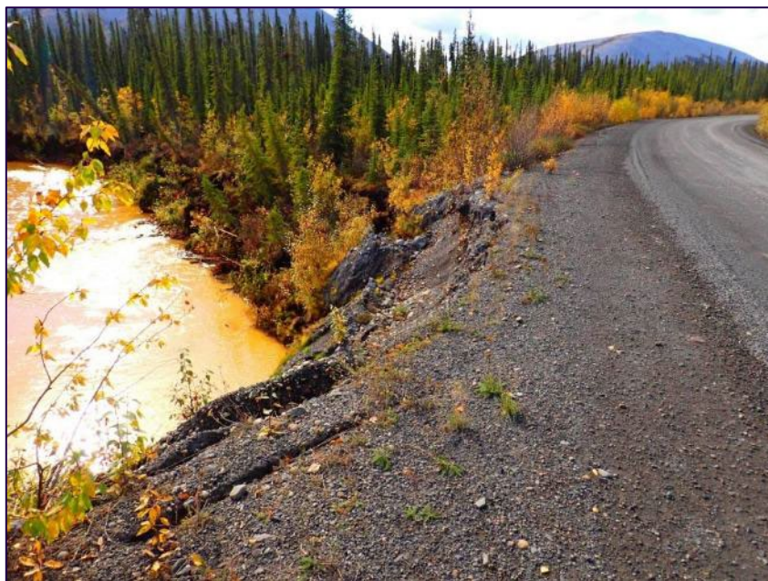
FIGURE 6.3. SCOUR UPSTREAM OF THE PREVIOUSLY PLACED RIPRAP AT DEMPSTER HIGHWAY KM 182.1
