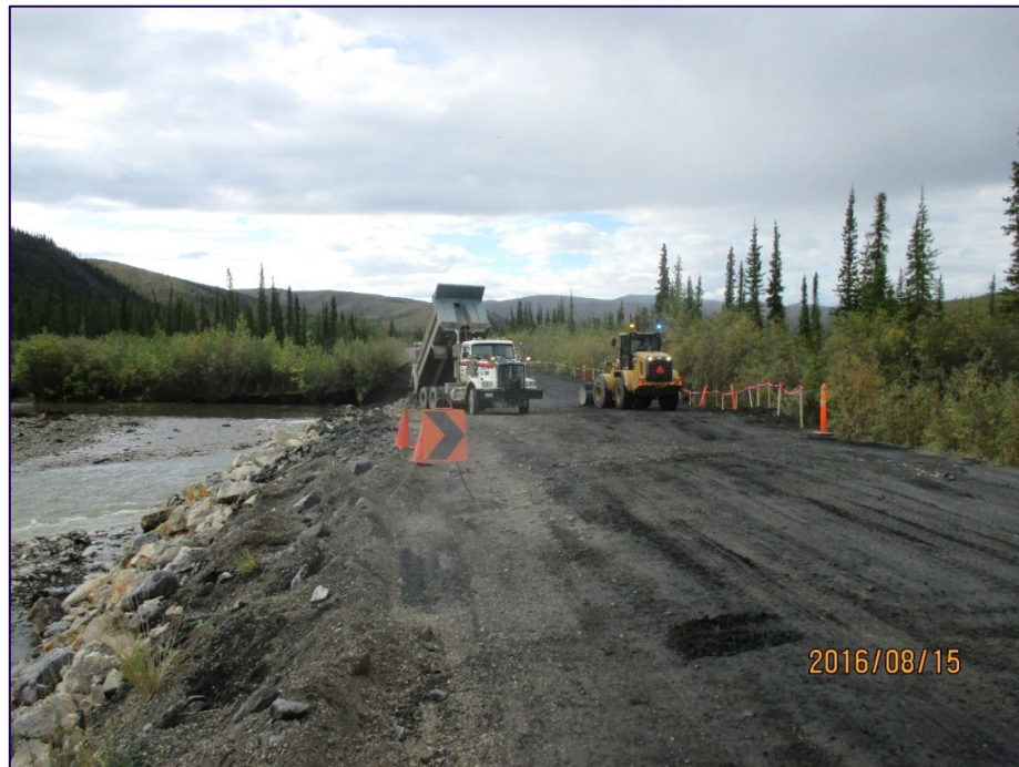
FIGURE 6.9. EMERGENCY RIPRAP INSTALLATION UTILIZING END-DUMPING METHODS FOLLOWING THE AUGUST 2016 FLOOD AT DEMPSTER HIGHWAY KM 165.5 (PHOTO CREDIT: HPW). WHILE EXPEDIENT FOR RAPID RESPONSE, THE LACK OF KEYED PLACEMENT AND MATERIAL SEGREGATION TYPICALLY RESULTS IN POOR STRUCTURAL INTERLOCKING AND LIMITED LONG-TERM RESILIENCE.
