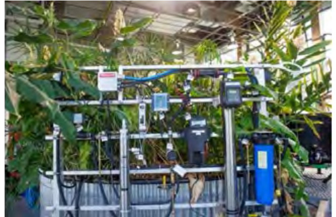
Figure 38 - Blackwater treatment at the Centre for Interactive Research on Sustainability at UBC
